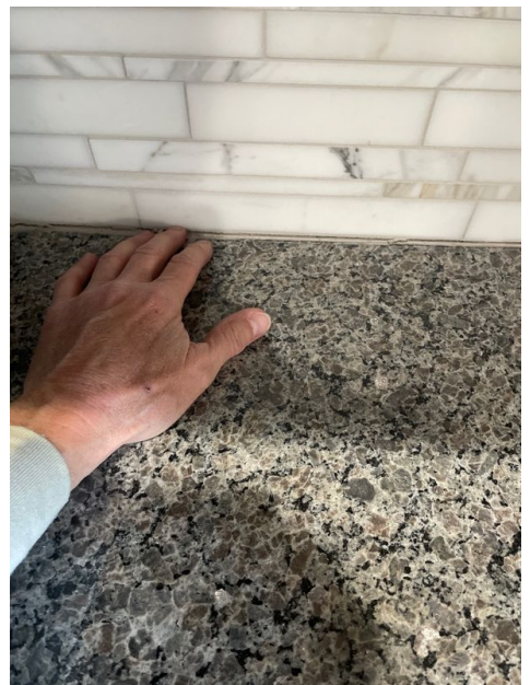
Kitchen Counter has Cracked Grout
